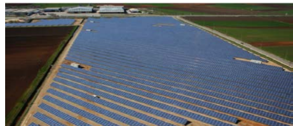
Picture 2-8 A PV power plant of 9.99MW peak , at Farsala Greece. Occupies an area of 34,900m 2 and consisted of 21,274 PV polycrystalline silicon modules.
