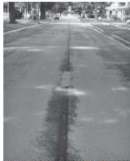
Longitudinal crack at joint
